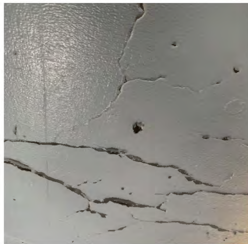
Figure 4: Failed SBS Spill Vault Coating
