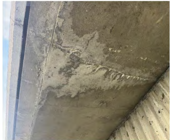
Figure 5: Signs of water seeping through walkway
