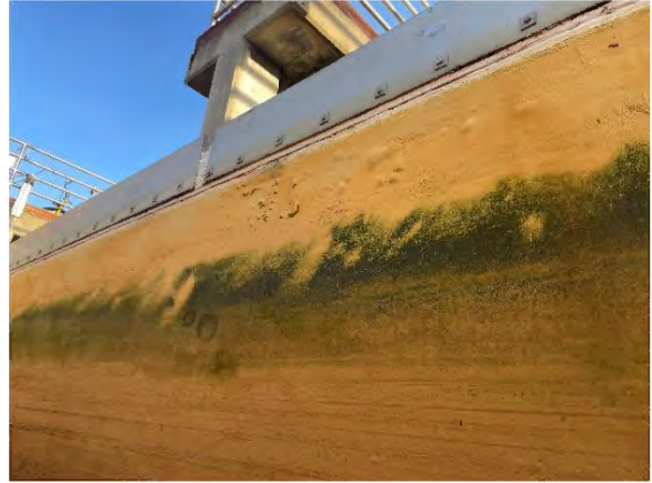
Figure 2: Failed Chlorine Contact Tank 4 coating
