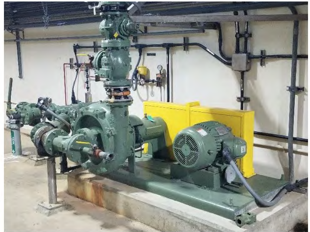
Existing Grit pump
